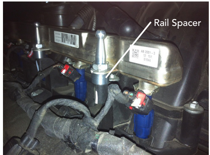
Fuel Rails Installed
