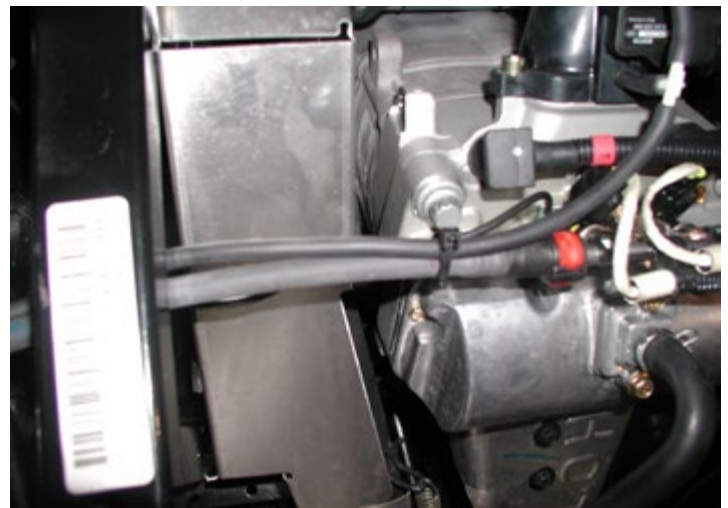
Vacuum Line and Wiring Routing
